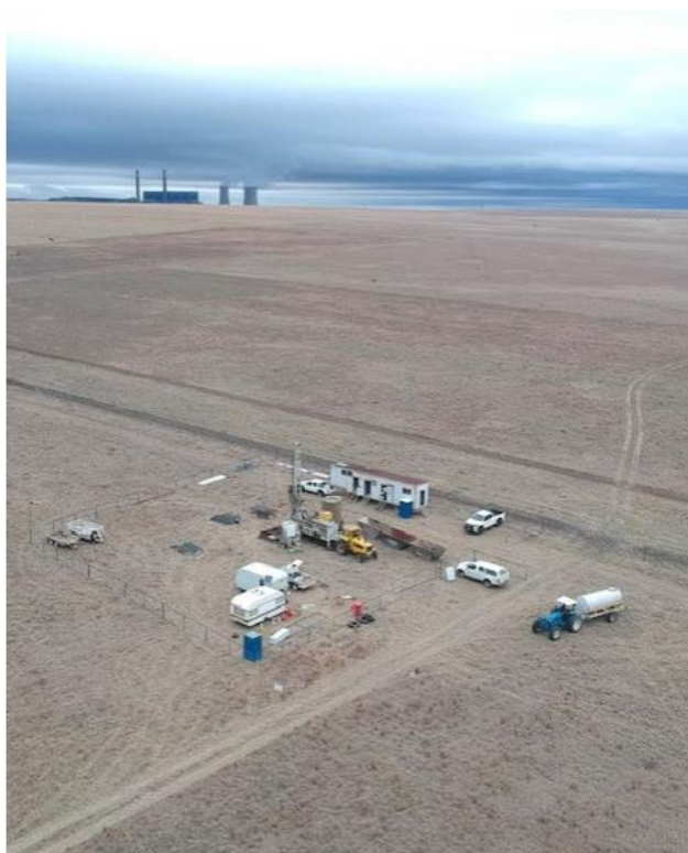
Exhibit 7 – Core well 271-23C being drilled with the Majuba power station in the background
